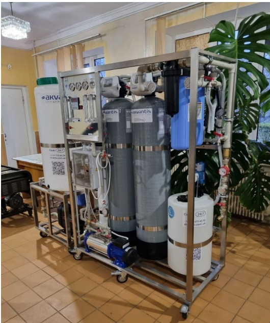
Figure 3: Image of first desalination plant, installed and operational in a hospital in Mykolaiv.
